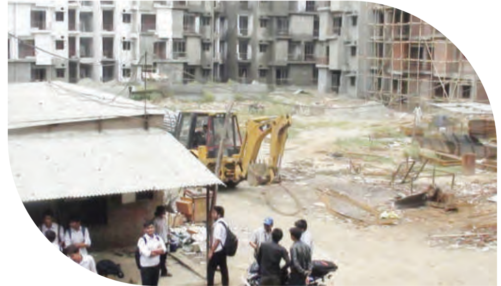
Industrial Visit to Brahmaputra Enclave, Siddhartha Vihar construction site was the part of Staad.pro Training for both batches. (Batch 1 & 2)
